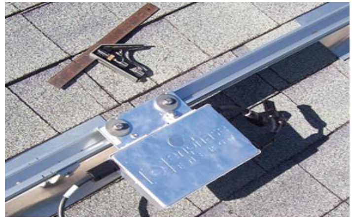
An Enphase microinverter mounted on racking. The PV module to which it attaches will sit right on top when the array is installed. Photo: Phillipsburg Electrical and Air.
